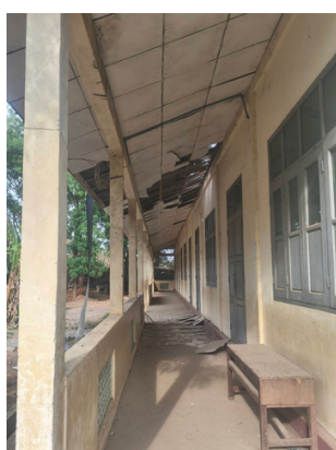
Documentation of damage to the school building in Htan Taw Kone Village, Chaung-U Township, Monywa District, Sagaing Region, caused by an airstrike on 16 May 2026.
